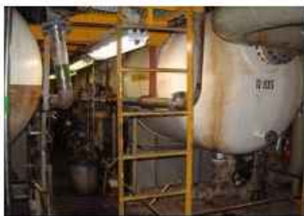
A test separator
