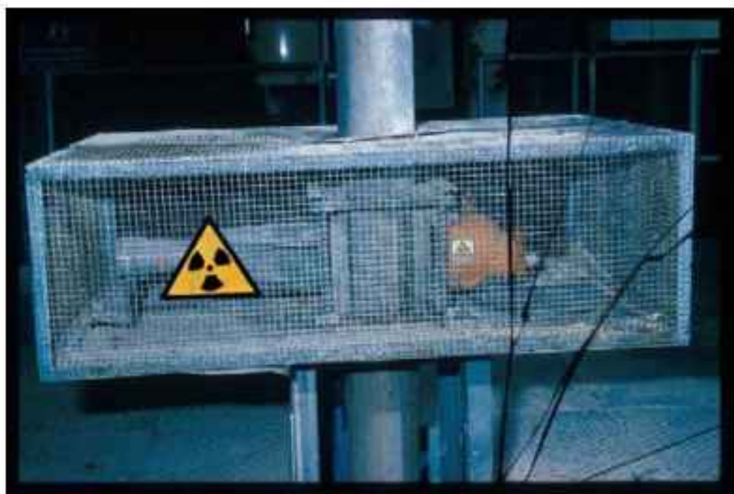
FIG. 15. Installed density gauge (Courtesy: HPA-RPD, UK)
