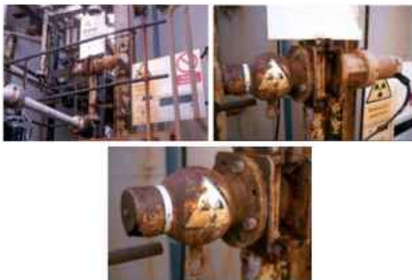
FIG. 76. Weathered nuclear gauge
